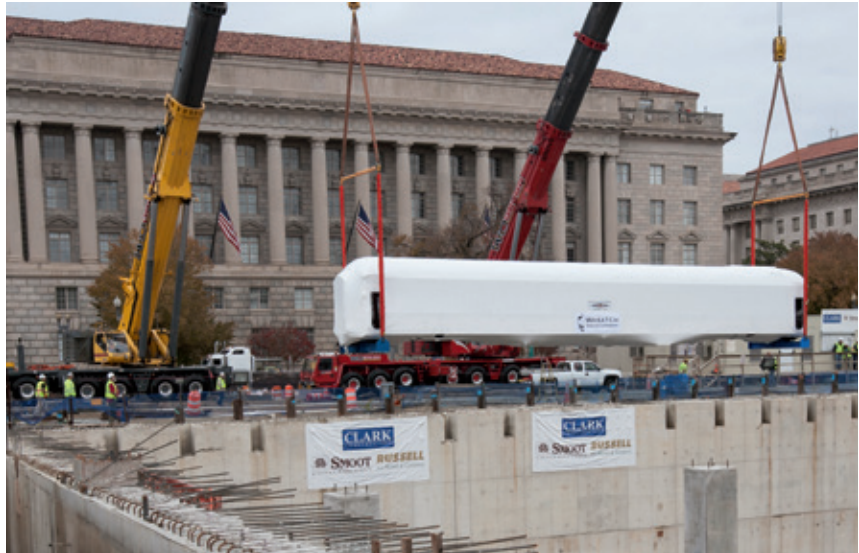
Two Grove GMK7550s place a railway car into the museum's construction site, an operation that requires careful planning and flawless execution.
