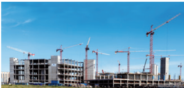
Potain tower cranes lift formwork, rebar, structural components, scaffolding and façade materials at the job site.
