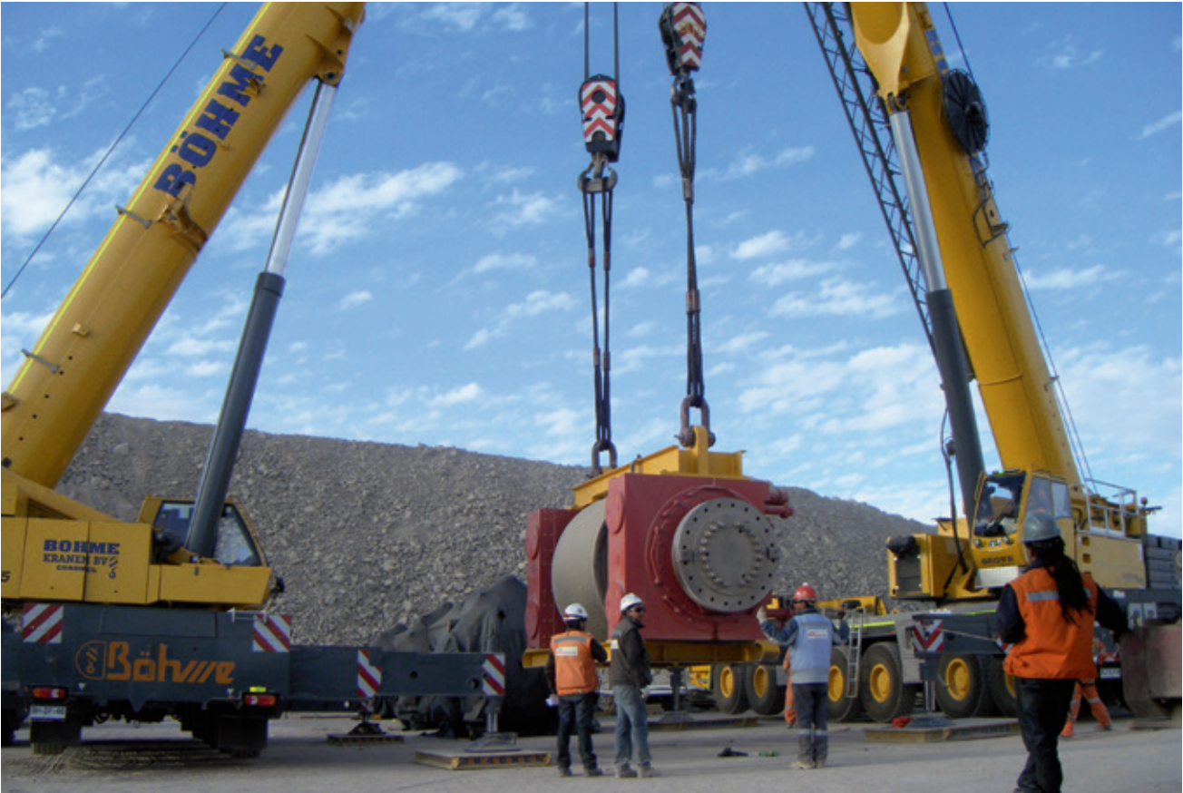
A 220 t (275 USt) GMK5220 and a 300 t (350 USt) GMK6300L jointly lift structural parts to prepare the site for production.
