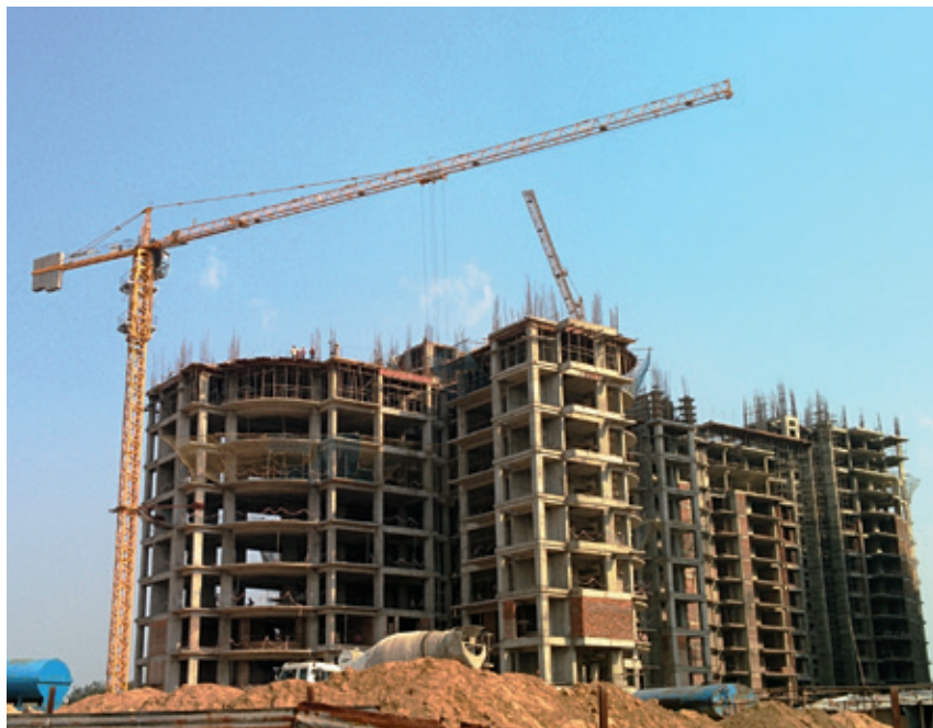
The recently refurbished Potain MCI 85 A tower crane works on a residential project in Gurgaon, India, soon after leaving Manitowoc Crane Care's facility in Pune.
