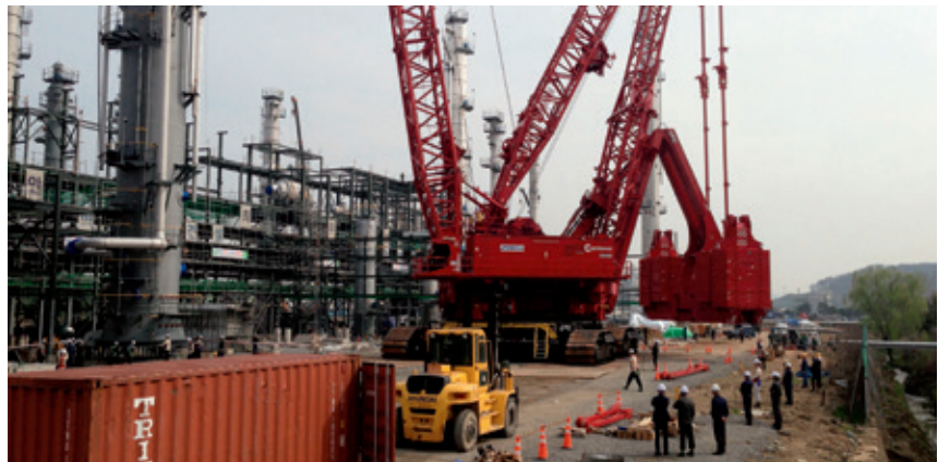
A Manitowoc 31000 lifts a 92 m (302 ft) tall wash tower that weighed 670 t (740 USt) with just 15 m (49 ft) of space for the counterweight.
