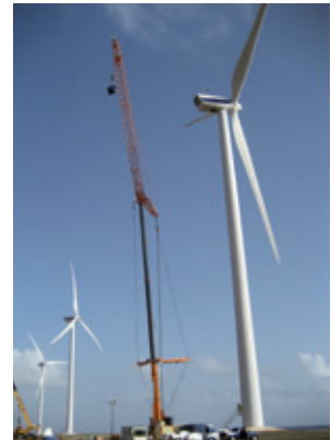
The GMK6400 performs maintenance at windmills up to heights of 80 m (263 ft).
