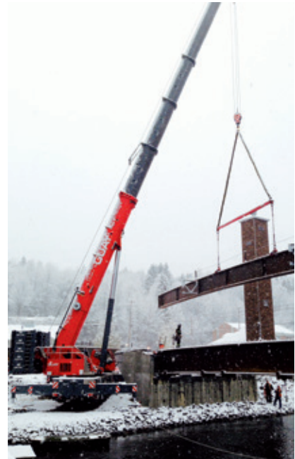
Guay uses its Grove GMK6400 to lift a bridge girder at Rivière-à-Pierre.
