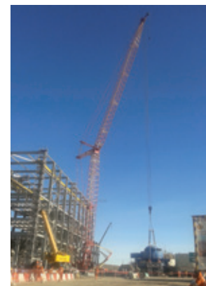
Rough-terrain cranes assist with the assembly of the processing facilities at a Peruvian mine.
