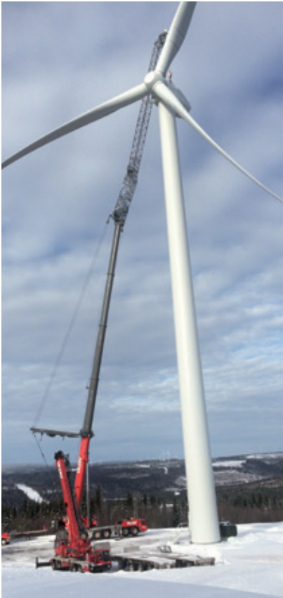
The Grove GMK6400 overcomes icy weather to erect a wind turbine in Lac-Alfred.
